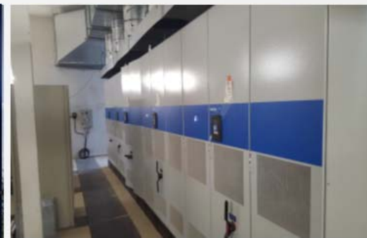
Vacon LHD in France (Water & Wastewater)
