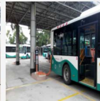
Zhongyeda China (Charging station)
