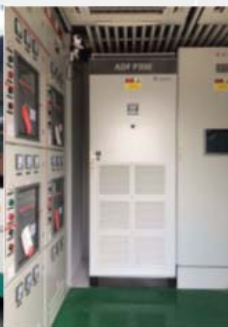
Zhongyeda China (Charging station)
